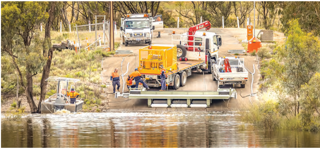
The relocation of the Waikerie ferry to its higher landing last week took about six hours to complete. PHOTO: Paul McCormick
