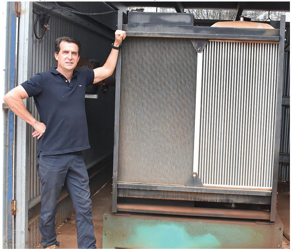
Omega Orchards owner Drew Martin with one of the large-capacity generators installed at his Murtho almond farm. Electricity supplies to Mr Martin’s irrigation pumps is at risk due to the current River Murray flood event. PHOTO: Hugh Schuitemaker
