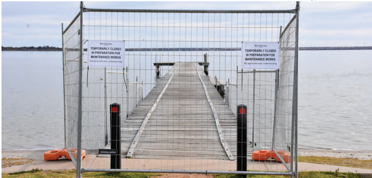
OFF LIMITS: Berri Barmera Council closed the Barmera jetty to the public last week. The council says it will remain off limits until it is stabilised. PHOTO: Peta-Marie Philippou
