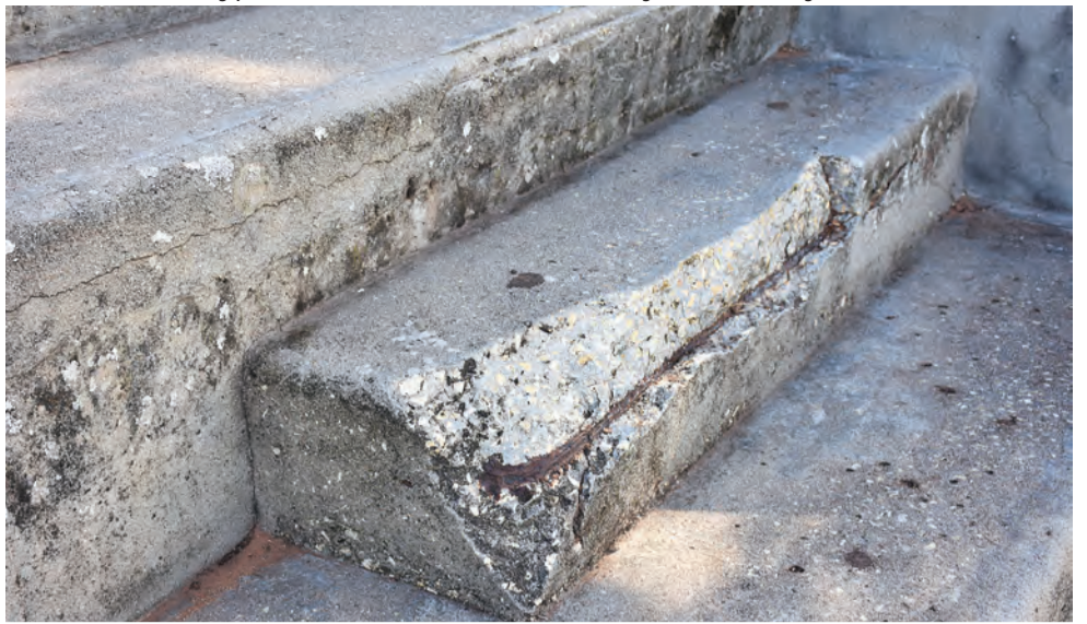
One of several concerns Mr Moritz has about the Berri wharf was the deteriorating state of the concrete swimming steps, which he believes are “not sound”. PHOTOS: Madison Eastmond
