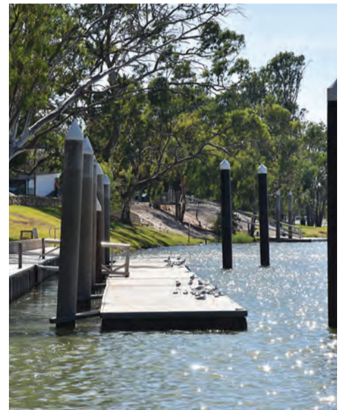
Without ladders available at the wharf, Mr Moritz said the “almost 1m” distance from the concrete edge to the water would be almost impossible for someone to pull themselves back up onto.
