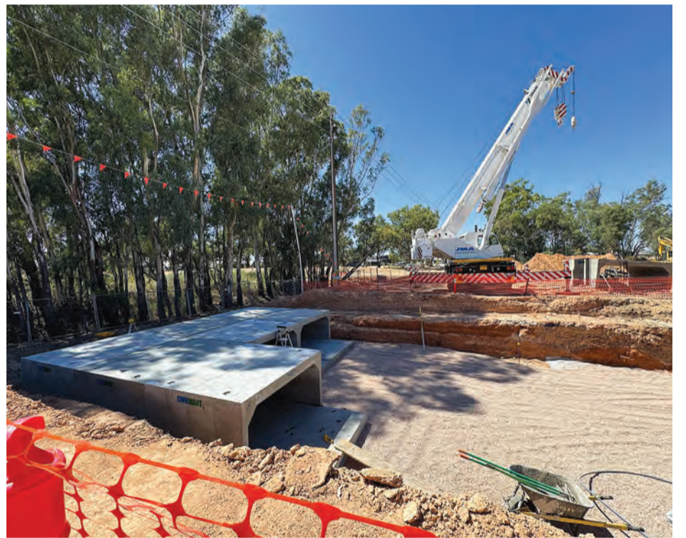
PROJECT UPDATE: The Twentyfirst street Bridge replacement is tracking well, with BMD Construction co-ordinating the final culvert installations happening in the coming weeks. PHOTO: Renmark Paringa Council
