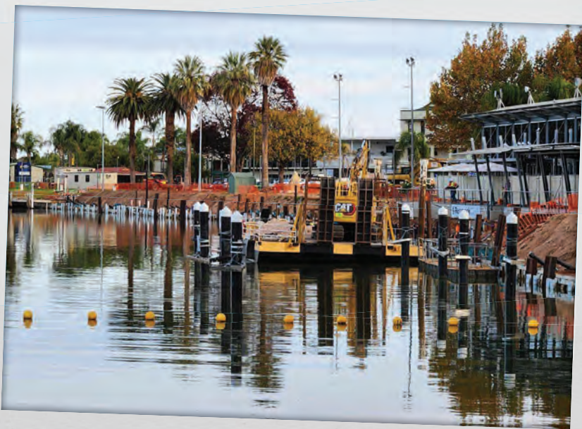
Works being done in May as part of a major redevelopment of the Renmark riverfront wharf.
